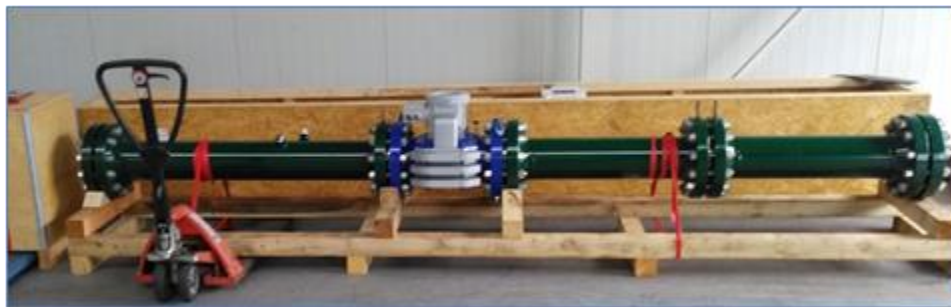
Figure 8: Complete USM package including flow conditioner (Source: GRTgaz)
