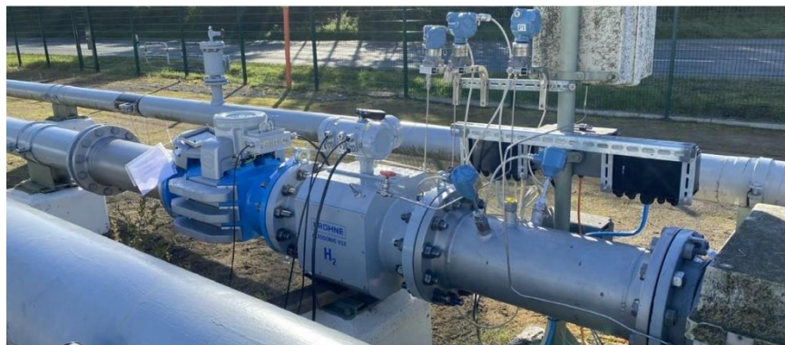
Figure 1: Test in Germany with UFM and TM in series on a 20 bar H 2 pipeline (Source: OGE and Evonik)
